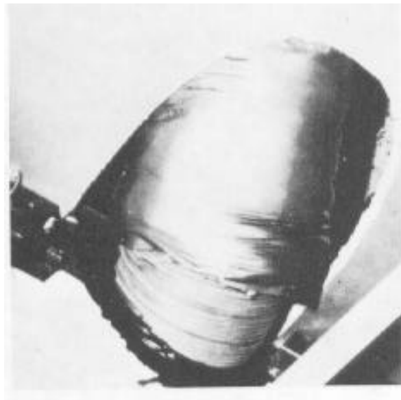
A fire-resistant ceiling is not effective if an architect or a workman allows wide holes for a pipe to pass through,
